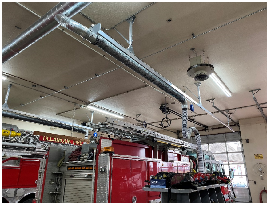
Image 8: Unbraced Duct in Apparatus Bay
