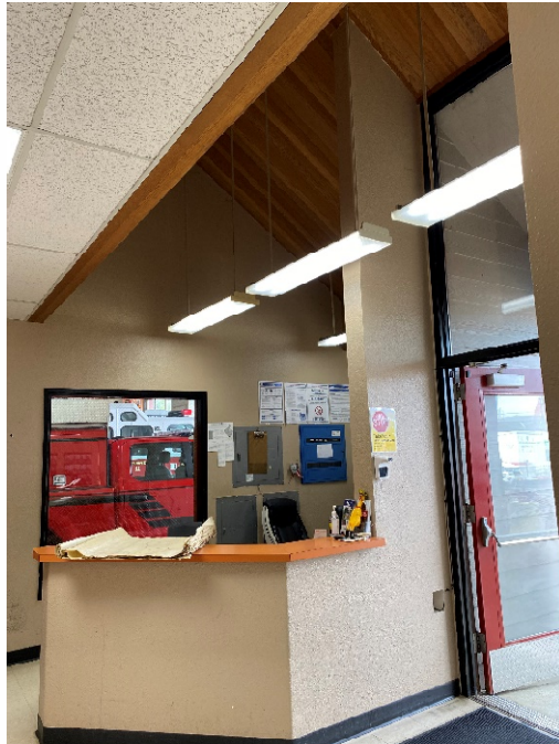
Image 5: Main Entry with Unbraced Lighting & Glazing
