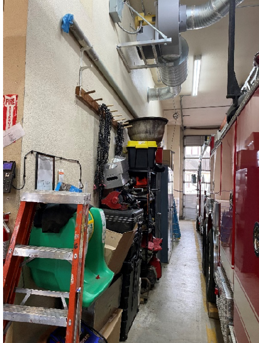
Image 10: Unbraced Cabinets & Shelving
